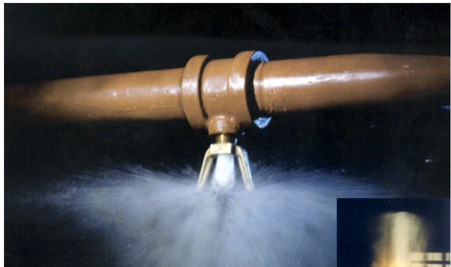
ESFR sprinklers in operation
